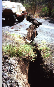
Photograph by Peter Lipman, USGS. Crack in Hilina Pali road, Hawaii Volcanoes National Park. Source: USGS HVO
