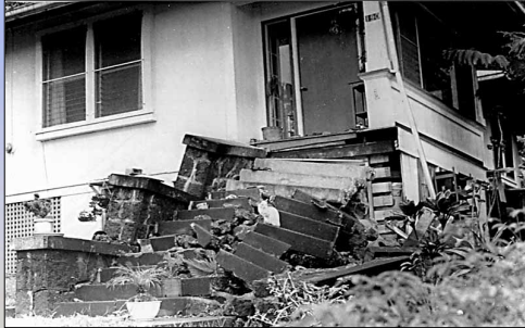
Photograph by UPI. Two children were trapped in this damaged home about 4.5 miles (7 km) north of Hilo. Source: USGS HVO
